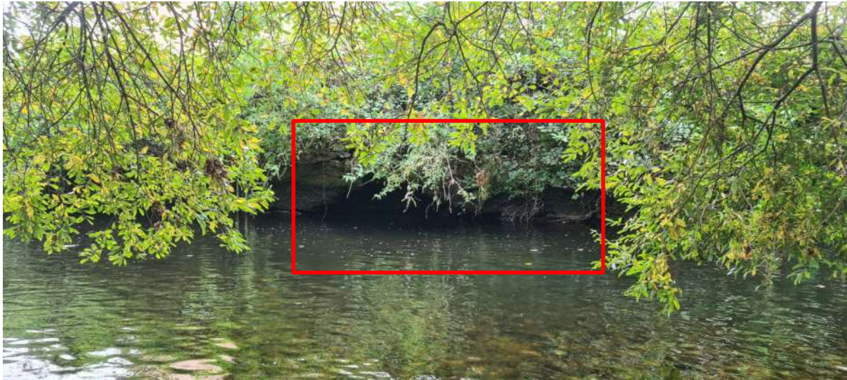
Figure 1: There is a significant void at the base of the riverbank retaining wall requiring remediation (red rectangle). The void in the face of the retaining wall void measures c. 3.5m long and extends c. 1.0m below the water line to the base of the wall and c. 2.1m from the external face of the walling back under the road above, creating a cave like structure. The ecologist was able to access the interior of the void and search for bats/ evidence of. The ecologist also searched other accessible roost features, and potential otter holts, hovers and rest sites for signs of otter.
