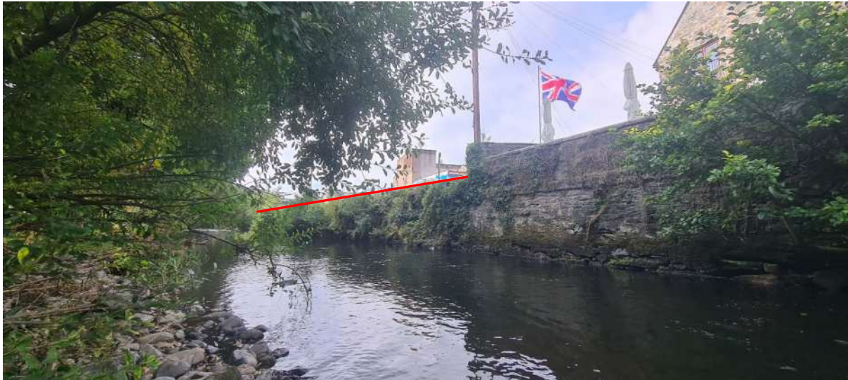
Figure 3: Section of wall requiring remediation works (red line); view southwest.
