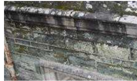
The exterior walls were mostly local Hurdwick stone, which is very porous and had decayed in places. Pointing has been poorly maintained using cement in places, which increased moisture ingress through capillary action.
