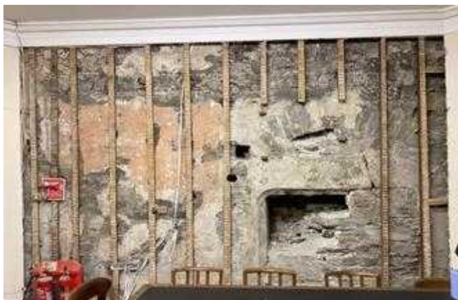
The medieval fireplace discovery where a new door opening was planned was both extraordinary and expensive! Archaeologists and Conservation Officer contributed to the strategy to retain this, necessitating the doorway relocation.
