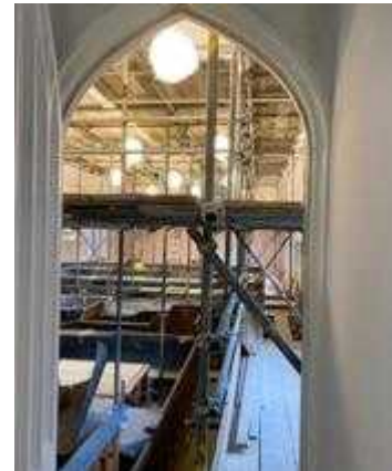
Scaffolding and access platform inside the courtroom to enable all new plastering to the walls. The joinery is protected beneath.
