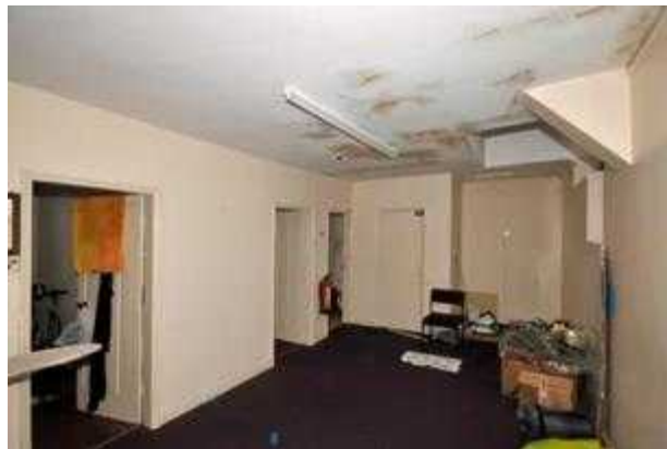
Water can be seen coming through the ceiling. Damp penetration entered either through junctions of the roofs, through the parapet walls and through the deterioration of the stonework forming the external walls.
