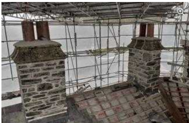
Joints were cleaned and repointed following discussion with the Architect and Conservation Officer after a lime mortar sample had been confirmed.
