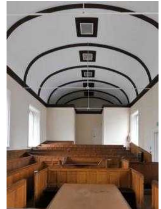
The 2 rooms seen here at the rear of the Magistrates Court were removed during the build works to make a learning space platform. This also greatly increased the light into the space.
