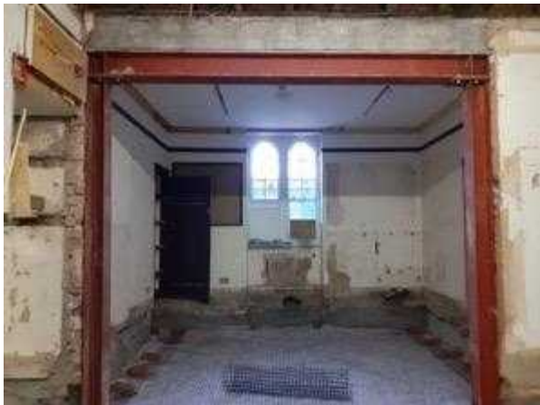
Openings had to be widened with steelwork to enable a workable visitor route and larger spaces for the new use.
