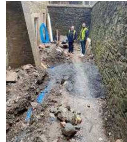
The new gas supply trench. Connecting to gas by Wales and West was a significant and frustrating delay of 7 months which created mould issues during decoration
