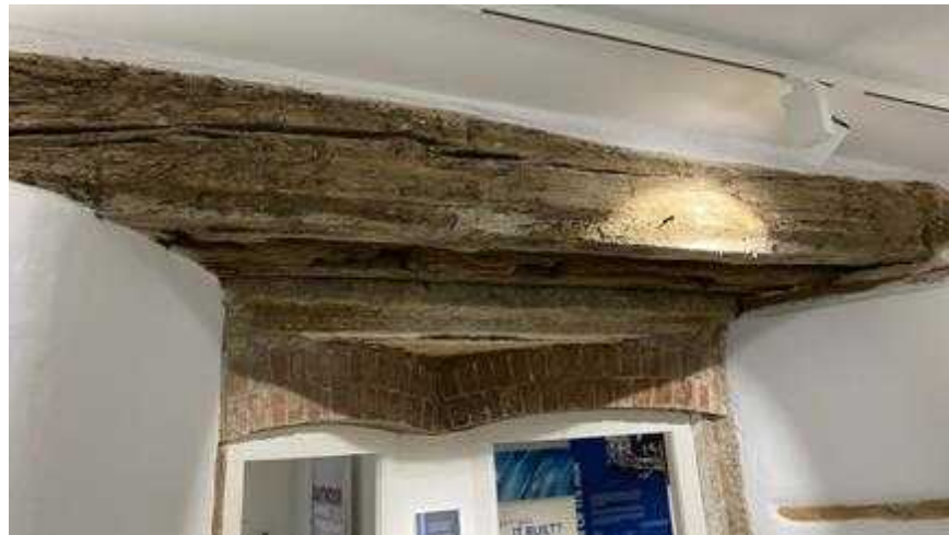
Historic fabric has been retained and featured such as these beams. Minimalistic exhibition lighting has also been installed.
