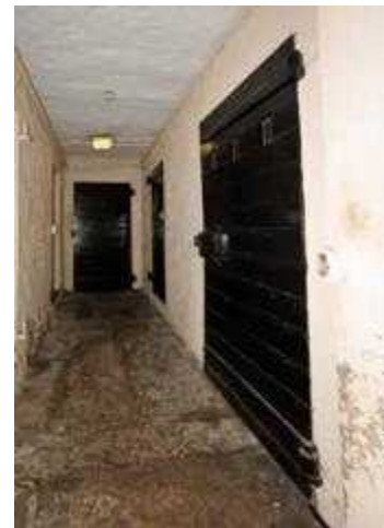
Gloss paint in the cells was trapping moisture. A general lack of repair and maintenance to the property had taken its toll.
