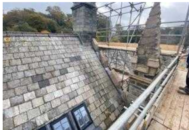
The original roof slates were retained, keeping the patina (not on Magistrates Court). RM Builders helpfully had a small supply of slates to help replace any that were broken. New roof lights were also installed.
