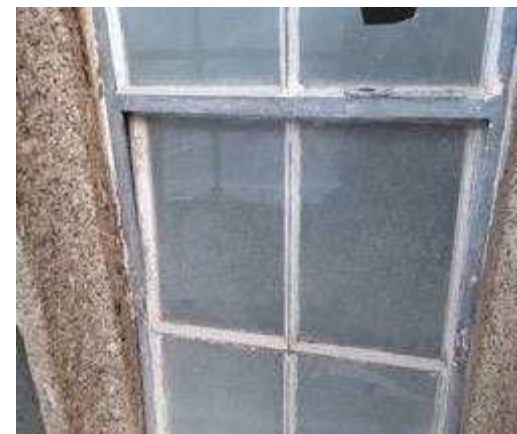
Window repairs underway, burnt off and prepared, putties redone. Replacement timbers came from joiners when required, as the building has a mix of timber framed double-hung sash windows and single glazed metal framed windows.
