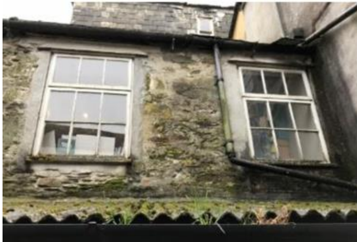
Sash windows in urgent need of repair
