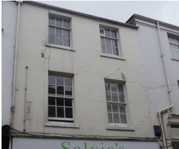
Before: Unsightly cracked render on the front elevation.
