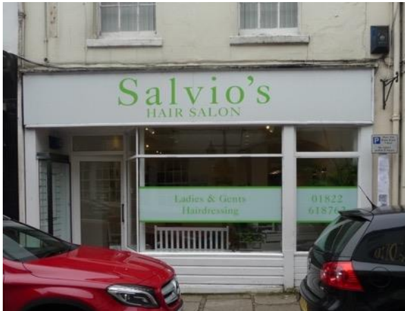
The above modern wooden panels were removed from the stall riser and replaced with cement board and render, with chamfered based.
