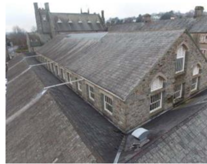
Before: Unsightly flying downpipes on the Pannier Market roof
