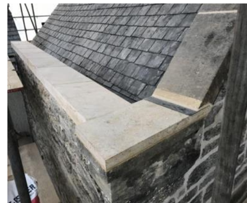
After: To improve the longevity and the aesthetic continuity of the building, concrete was replaced with Ham Stone rather than replaced like for like. It proved to be much the same cost.
