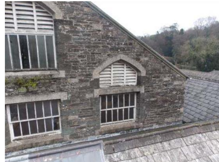
Before: The extensive windows required overhaul and repair, including piecing in timber to sills which had suffered decay. The gable end louvered openings were a source of heat loss.
