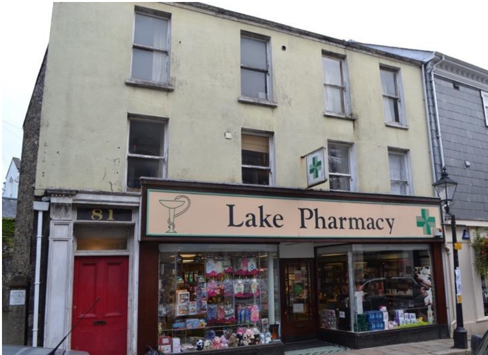
Before: In a poor condition. The oversized fascia did nothing to enhance the Conservation Area.
