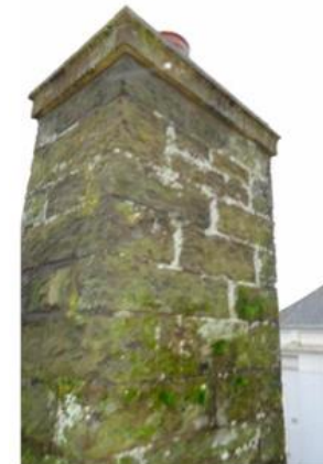
Before: Saturated stonework from cement pointing
