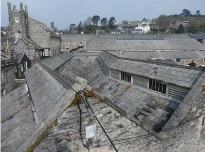
Before: Insufficient maintenance led to the poor roof condition.
