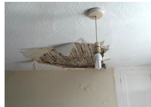
Water used to leak through the roof into bedrooms, and a piece of ceiling had falling down.
