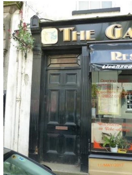
The shopfront in a poor condition. The Dutch blind above the shopfront installed without LBC was removed as a condition of the funding.
