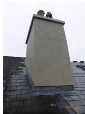
The project enabled both properties (9 and 10 West Street) to benefit from a fully repaired and rendered shared chimney, which was not previously feasible to do.
