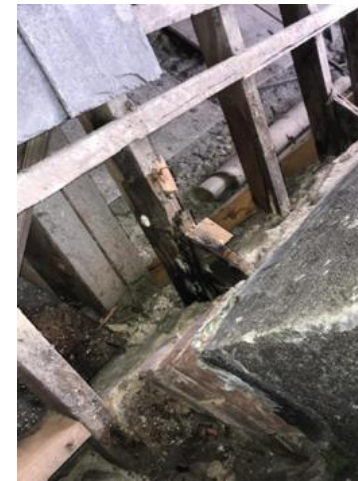
The replacement of original parapet lead lined valleys with mastic asphalt had degraded, resulting in significant water ingress and decayed underlying timber formwork and rafter ends.
