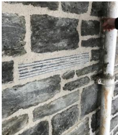
SPAB style repairs were undertaken where wall stones had fully degraded, using length of Delabole slate bedded horizontally in lime mortar.
