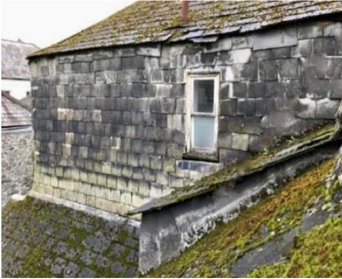
Before: Natural and fibre-cement slates in poor condition
