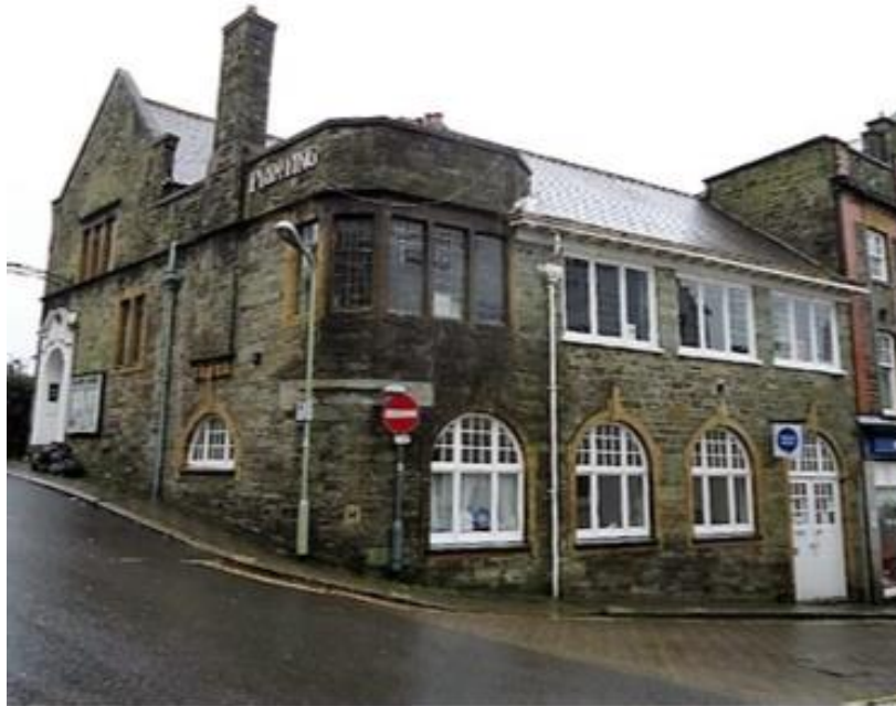
Before: Original signage had been partially removed without Listed Building Consent.
