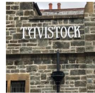
Decayed signage removed and faithfully reinstated on 'The Printworks', formerly Kingdon House.
