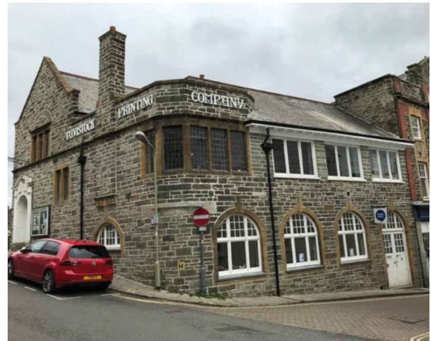
After: The outside of the buildings looks almost as it was in 1907, with repointing, reinstated rainwater goods and signage.
