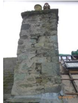
Before: The shared chimney was in very poor condition, and stones had previously come lose and fallen.
