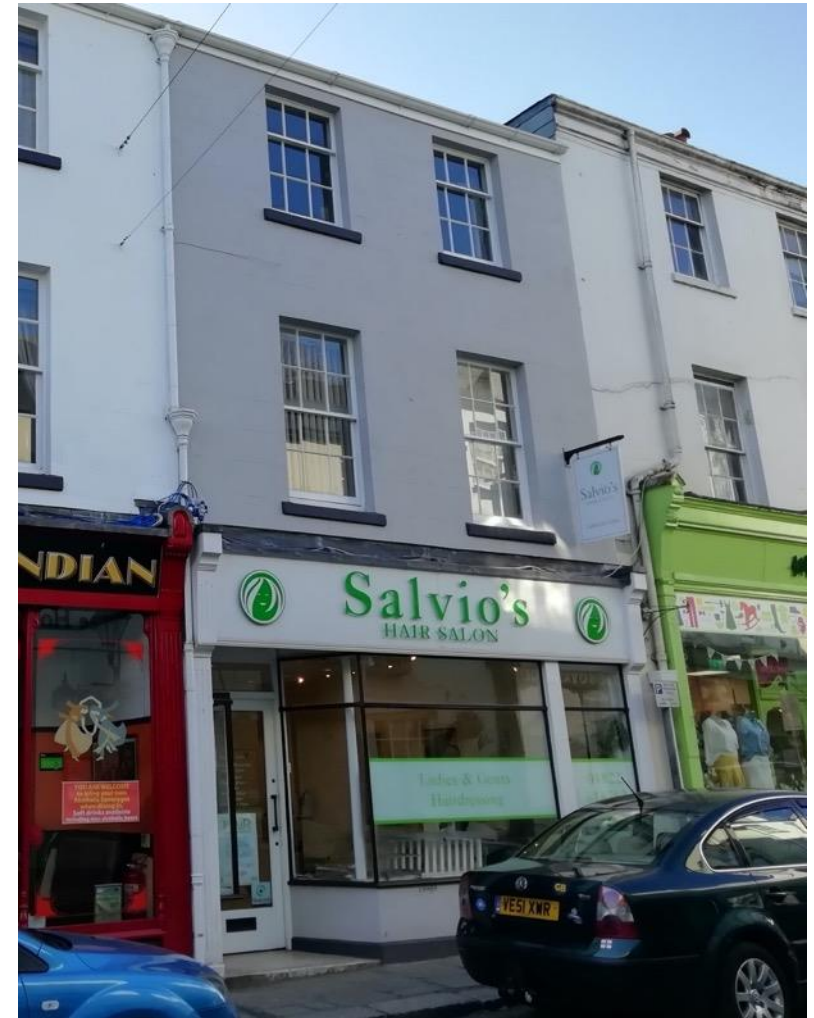
After: The reinstatement work on the shopfront included forming new fluted pilasters and corbels, fascia and projecting the cornice with lead flashing.
