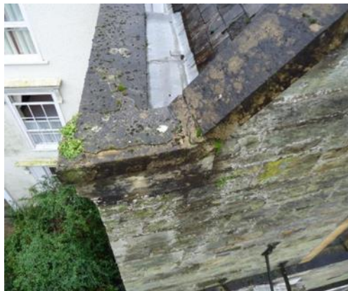
Before: Replacement cast concrete parapet coping stones were in poor condition.
