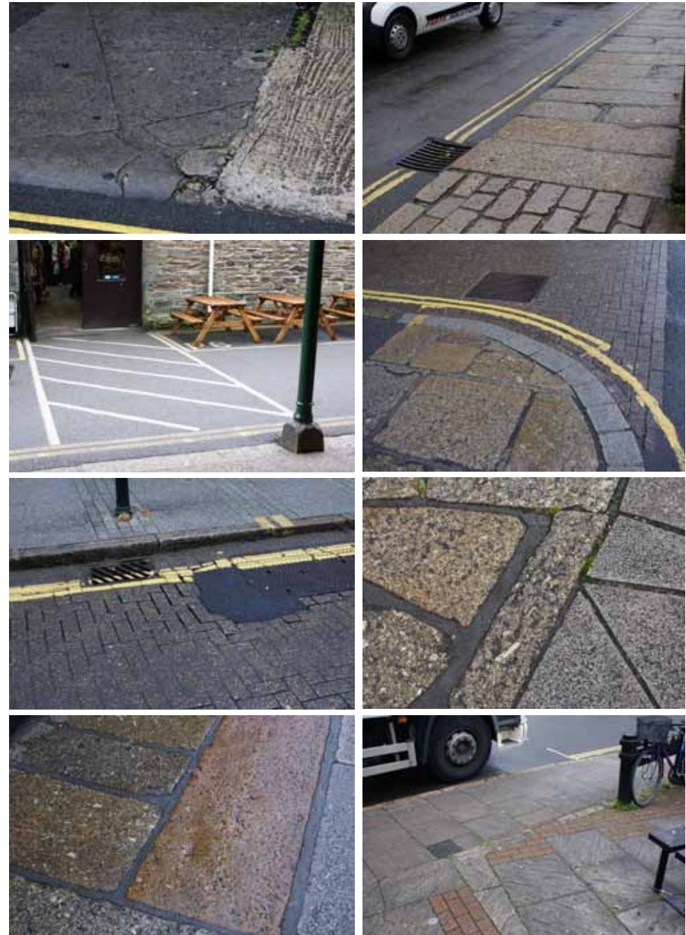
INCONSISTENCY IN PAVING
